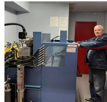
Regional Fire Dept SCBA Filing Station
